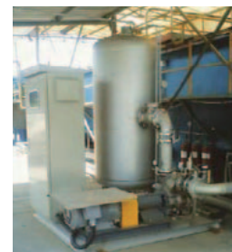
30-kW micro-bubble aerator at textile factory in Shanghai
