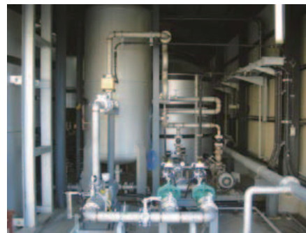
Pressurized flotation unit with processing rate of 35 m 3 /h
