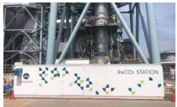
CO 2 recovery equipment (ReCO 2 STATION)
