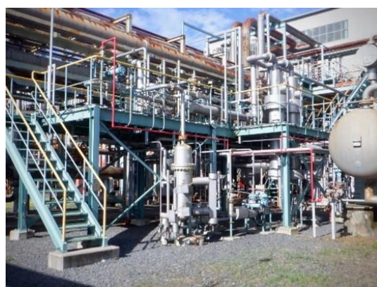
Hydrogen concentration system
