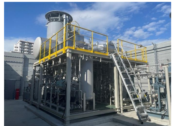
Hydrogen generator (VHR)
