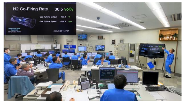
Central control room during a 30% hydrogen co-firing
