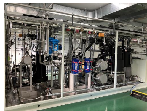
100kW fuel cell evaluation equipment
