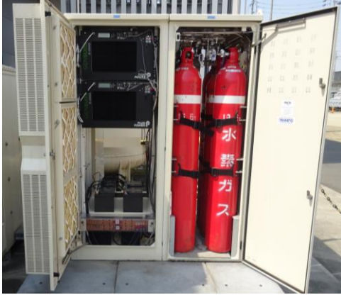
E-2500×2 5kW power generation fuel cell system
